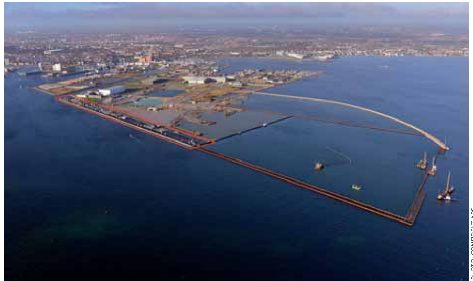
Work in November on the new port area including the cruise ship quay in Copenhagen, in operation Spring 2014.
